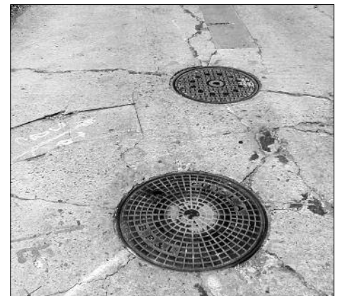
An underground electricity vault in Oaks, probably installed in the 1930's. B.P. & L. stands for "Bureau of Power and Lighting." The ground has quite visibly shifted over the years.
