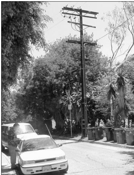
At the northern end of Phase 1 on Live Oak East, where the distribution line comes up from below.
